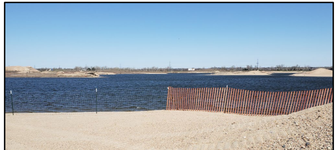
34 Woven wire and wood slat fence deployed on north 35 shore of Broadfoot South-Kearney. Top wire had not 36 been installed yet.
